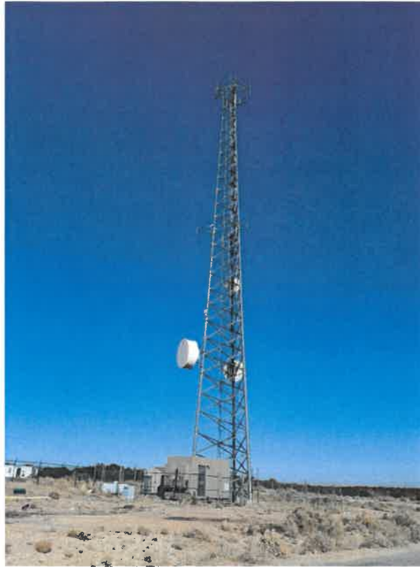
The NTUA tower showing the microwaves used to provide data to the casino and hotel and the space available for cell antennas at the top of the tower
